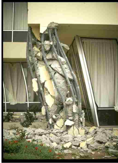
Figure 1.2 - Damaged column at Olive View Hospital, from [Steinbrugge 1992]
